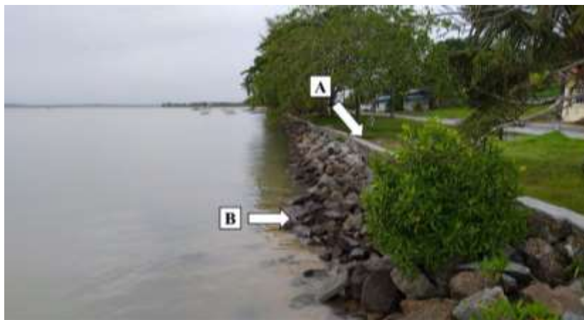
Figure 5. Wave breaker constructed along the beach to avoid beach erosion. A: Concrete wall. B: Stack of boulder.
